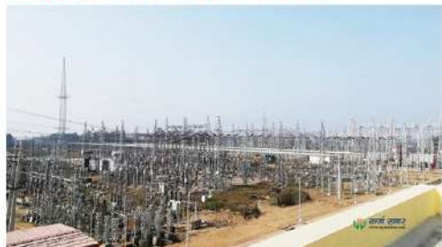
Figure 11.32: 400 kV Sub-station located at Dhanusha, Dhalkevar
